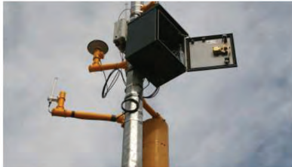
Figure 4. Roadside equipment at 36 th St and 11 th Ave, New York.
